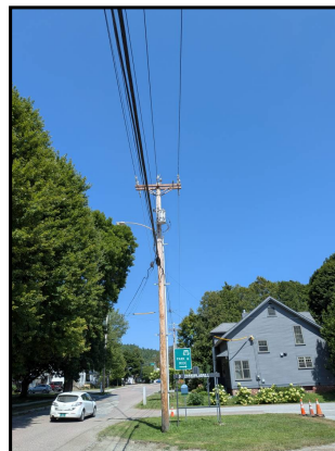
8: Pole mounted transformer with "Non-PCB" sticker
